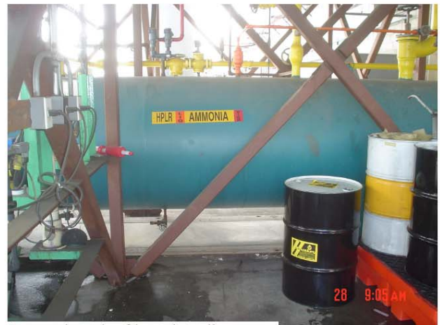
Ammonia and refrigeration oil
