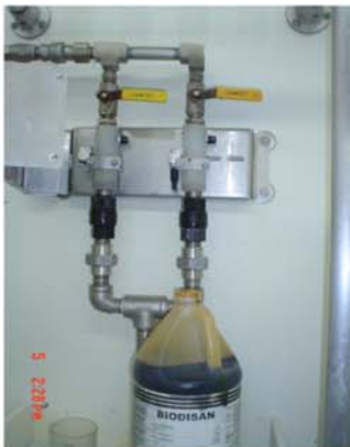
Chemical mixing valve
