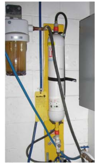
Water de-ionizer – battery filling
