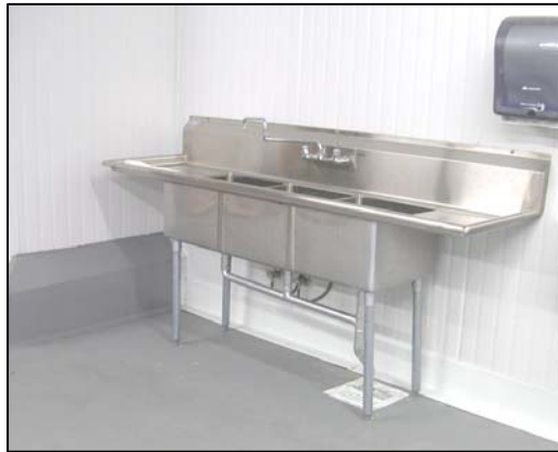
Photo 4 – Three compartment utensil wash sink
